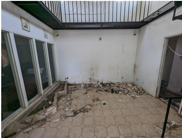
Debris throughout floor
